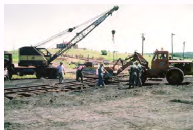
DM&IR workers laid temporary tracks up Clubhouse Hill to enable the move to take place.
