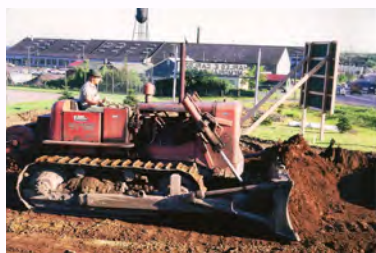
Prior to August 8, crews from the DM&IR's Track Department prepared the Clubhouse Hill site.
